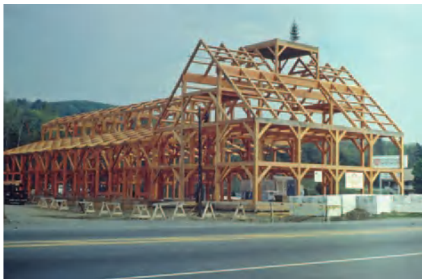
Figure 8 Diagonal braces lend rigidity to the timber frame of this future retail shop. Courtesy of Bensonwood Homes.
