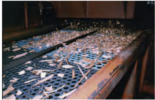
Figure 12 A typical gyratory screen. Note that the round holes are larger in the feed end of the screen and smaller at the discharge end. This has been used to increase screen capacity, but actually reduces removal efficiency.
