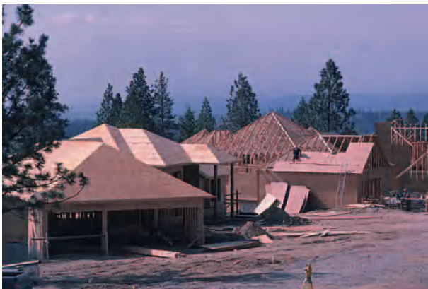
Figure 5 Light-frame buildings constructed from dimension lumber and plywood or oriented strand board sheathing such as these houses are the most common wood-frame structures. Courtesy of APA – The Engineered Wood Association.
