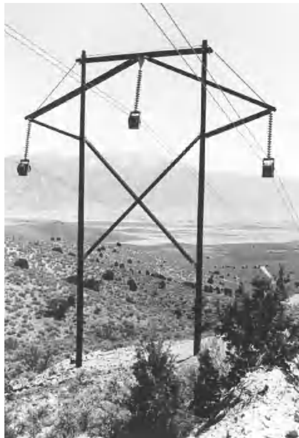
Figure 1 Round timber poles form the major structural element in these transmission structures. Courtesy of Koppers Co.
