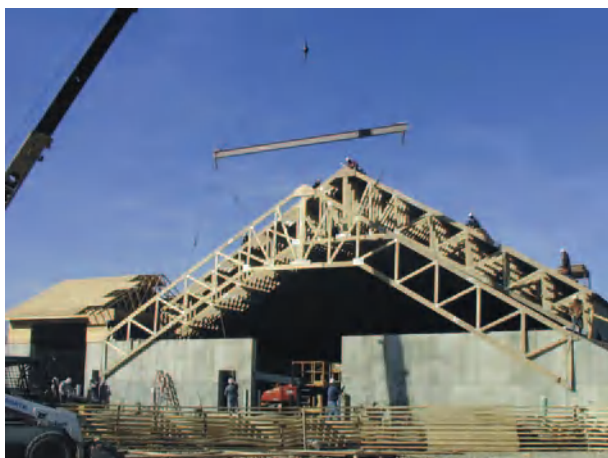
Figure 3 Roofs of virtually any shape can be framed with metal plate connected wood trusses fabricated from dimension lumber. Courtesy of the Wood Truss Council of America.
