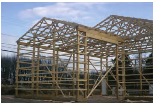
Figure 7 Diagonal bracing holds the dimension lumber walls and roof trusses of this post-frame building plumb and square before sheathing is applied. Courtesy of National Frame Builders Association.
